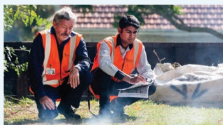
In some cases we use non-toxic smoke to pinpoint places where stormwater is entering our wastewater network – like the leaky pipe in the ground, pictured above.
